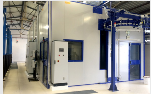
Paint booth - (CORELEC)
